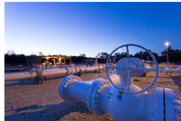
Southern Hills Pipeline
